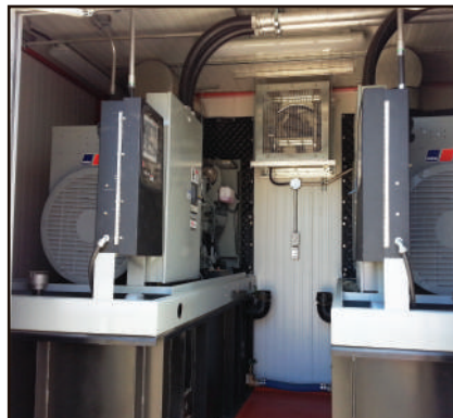
2x 125 kW Generators
